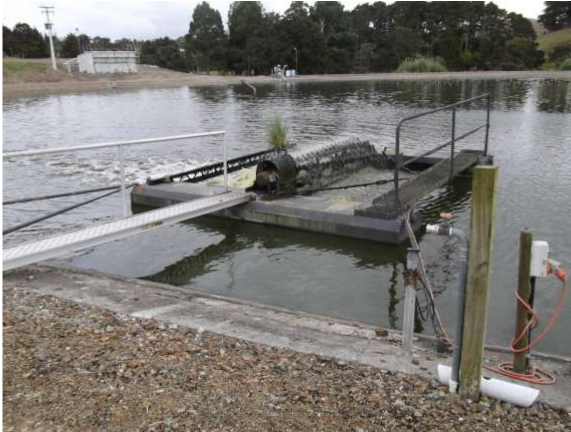
Figure 3-20 : Maungaturoto WWTP aerator
