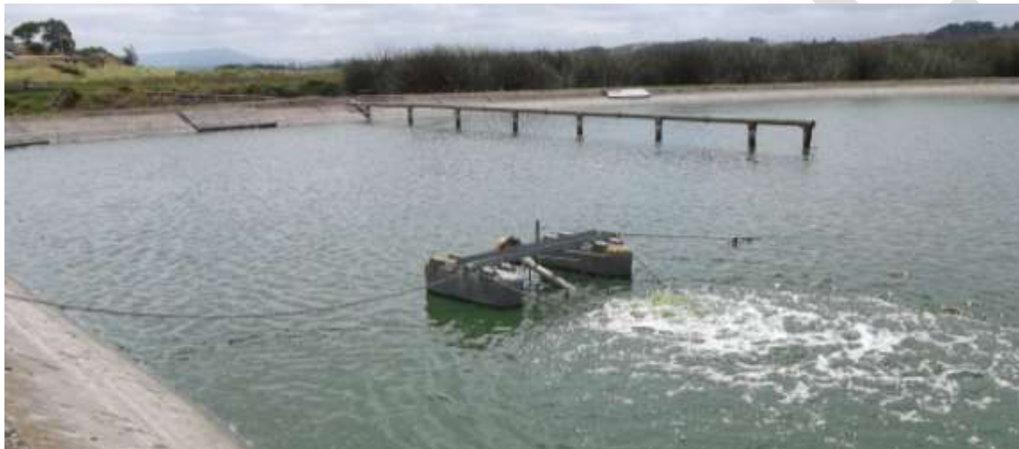
Figure 3-23 : Te Kopuru WWTP oxidation pond
